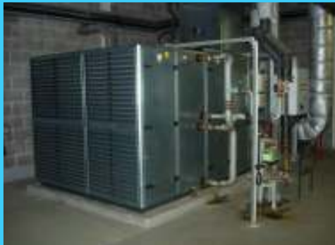
◀ Air handling unit installed at Swansea Bay.
